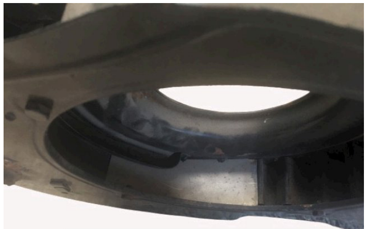
tin plate inserted into the top of the upside-down fan housing to block off heater channels, before welding
