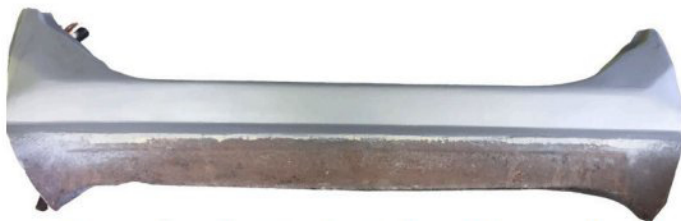
The bottom half: horribly pitted with rust. The top bit: lovely and smooth thanks to many applications of filler and abrasive paper.
