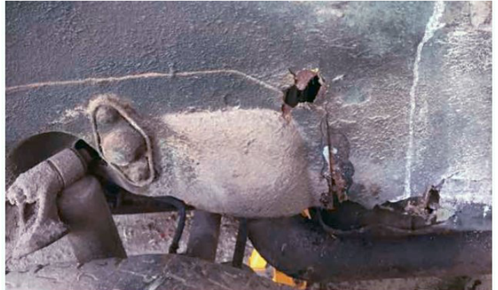
A good example of rust traps caused by reinforcement panels
