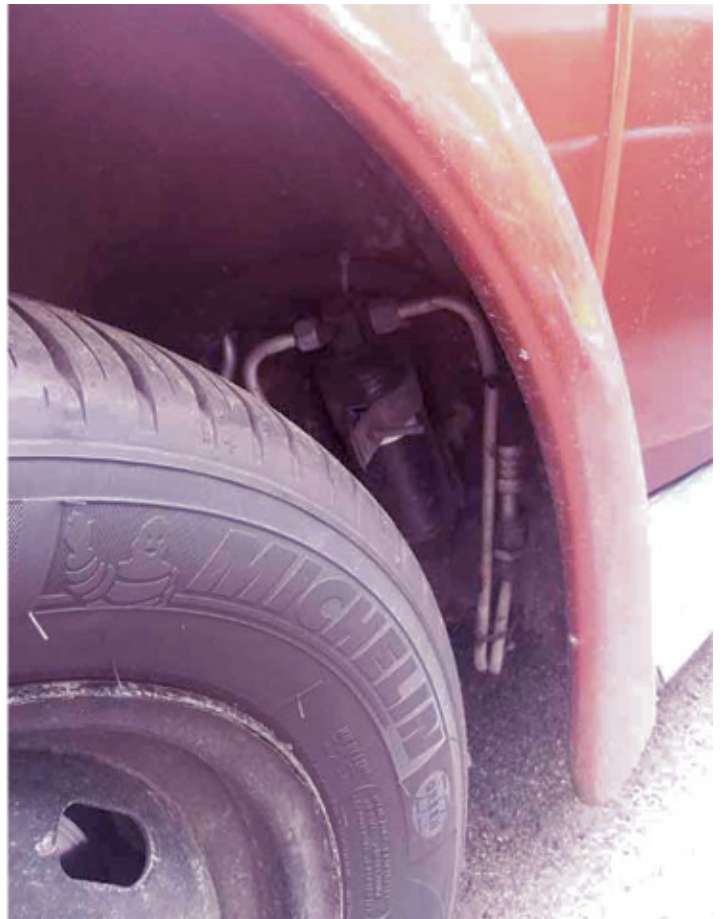
The receiver/drier is under the front LHS mudguard. That makes the sight glass a bit hard to see.
