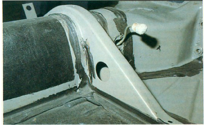
Original lhd chassis - no floor reinforcement on right-hand side. Note also master cylinder aperture provided in inner skin of bulkhead only; hole must be accurately replicated in outer skin, and spacers inserted to avoid distortion and movement.
